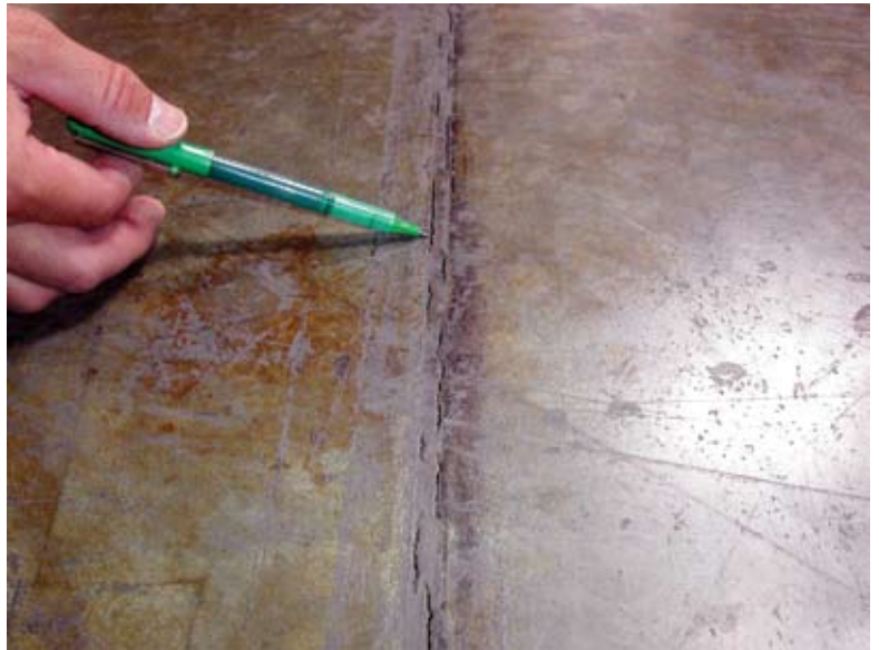
Epoxy separation after one year at new slab joint. Note that epoxy is still providing some protection of slab edge
