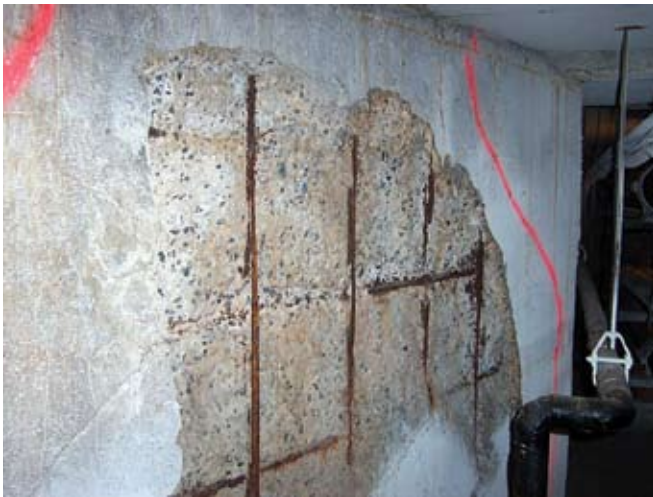
Fig. 4: Spalling and reinforcing steel corrosion in northwest diagonal wall. Note section loss in reinforcing steel
