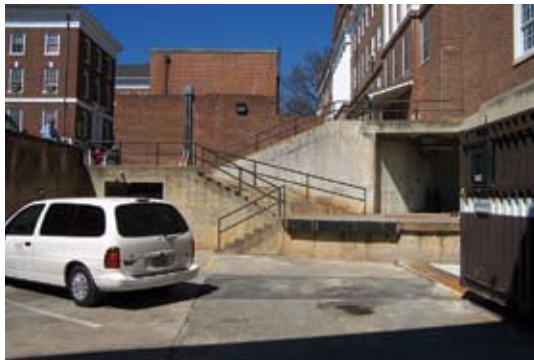
Fig. 1: Elevation view of loading dock, looking west, before restoration. The door to the steam tunnel is behind the car to the left
