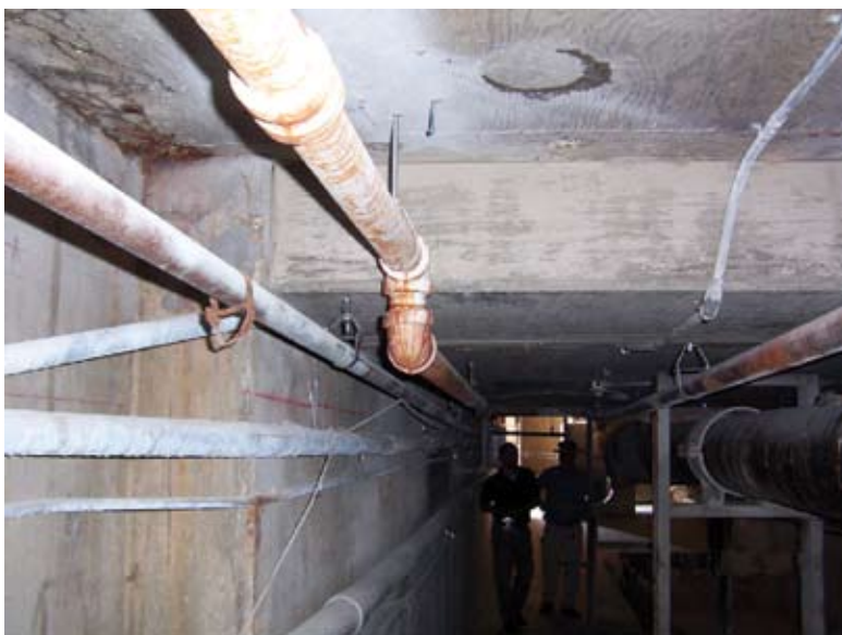
Fig. 9: Concrete beam after restoration (compare to Fig. 6)
