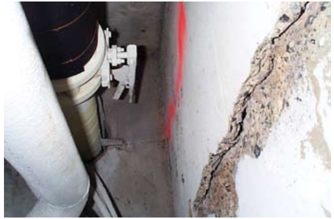
Fig. 5: Delamination, spalling, and scaling in the common wall between the steam tunnel and electrical manhole
