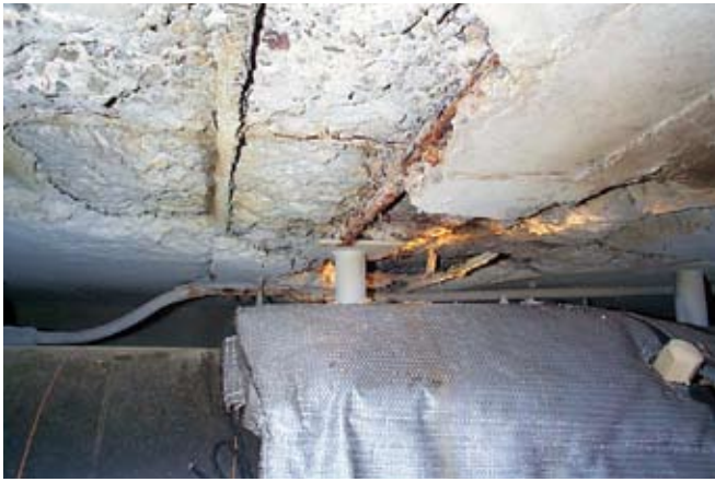
Fig. 3: Deterioration in the tunnel soffit
