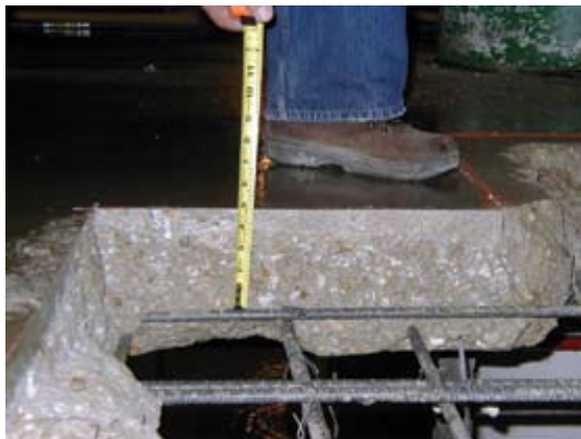
Top mat of reinforcing steel with 4-3/4 in. of cover. Note the top bar was actually tied to the bottom mat of steel
