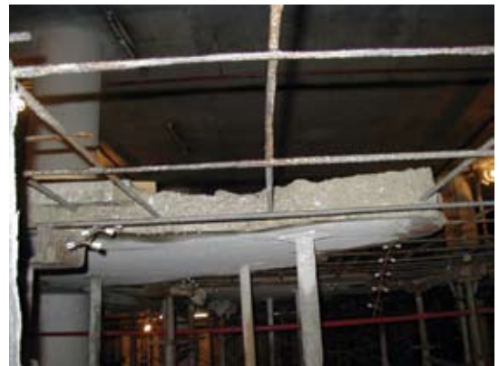
Full depth repair. Note the depth of the top mat located at the left side of the picture. The top mat is depressed to mid-depth of the slab
