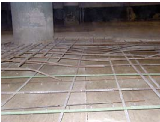
Full depth repair area. Note the deflected top bars, from original concrete pumping operations and additional epoxy coated bars were installed due to the lack of amount of bottom steel
