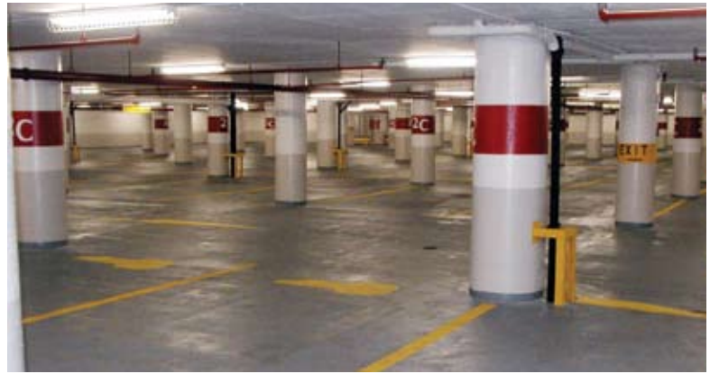
The finished garage. The battleship gray waterproofing membrane has sealed and protected the new repairs and original concrete from additional chlorides entering the slabs. The entire garage was painted and new lighting was installed
