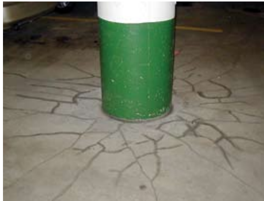
Typical top surface negative moment cracking around column due to low top surface steel location
