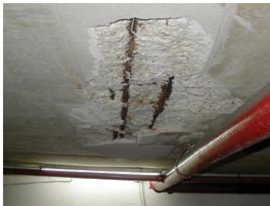
Typical previously repaired soffit patch. Note the old patch was not properly repaired—the reinforcing bars were not undercut
