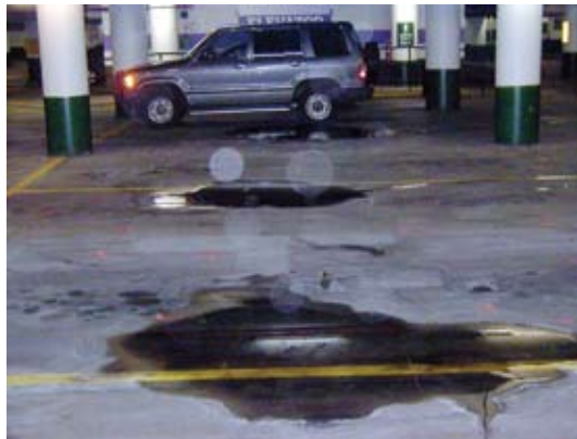
Typical ponding of water at low spot in center of bay
