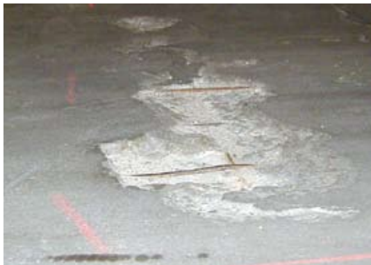
Typical top surface delamination with exposed reinforcing bars
