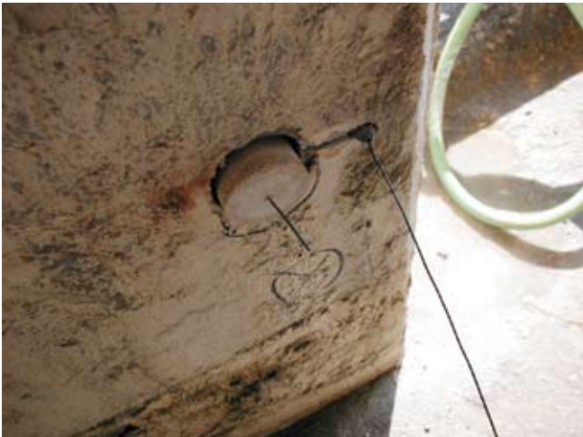
Close-up of anodes and reinforcing bar connector
