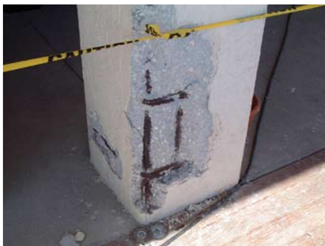
Typical concrete damage on ground floor columns
