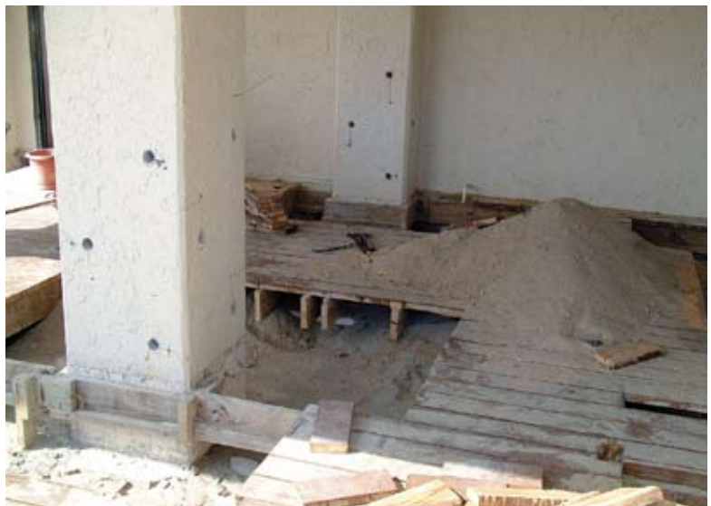
Decking removed and sand excavated for access to column below sand line
