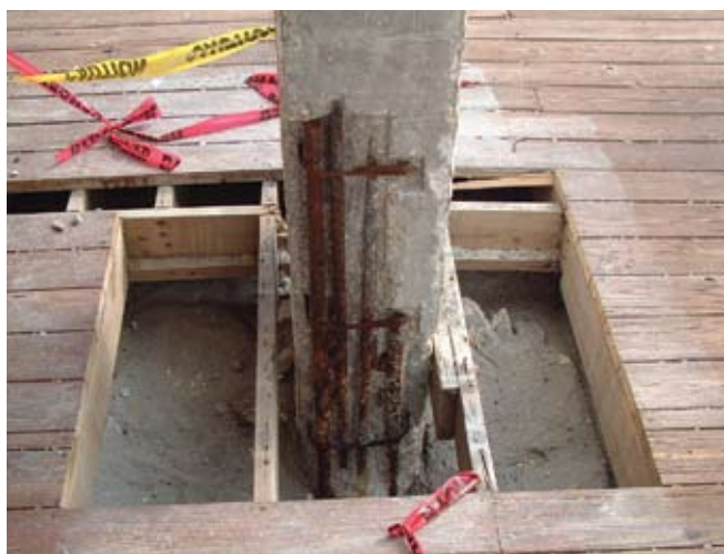
Significant concrete damage on 12 x 24 in. (30.5 x 61.0 cm) column
