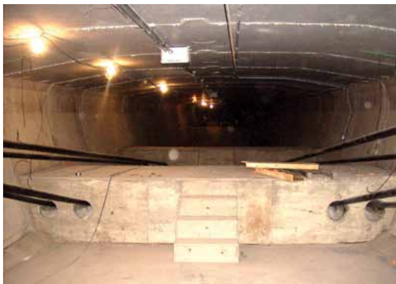
Installed tendon profiles
