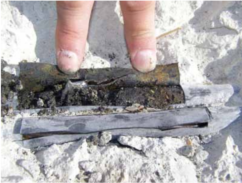
Fig. 5: Exposed strand with severe corrosion and wire section loss for a push-through system
