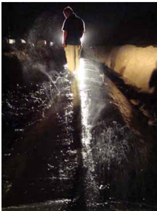
Fig. 2: Leaking after conventional crack sealing
