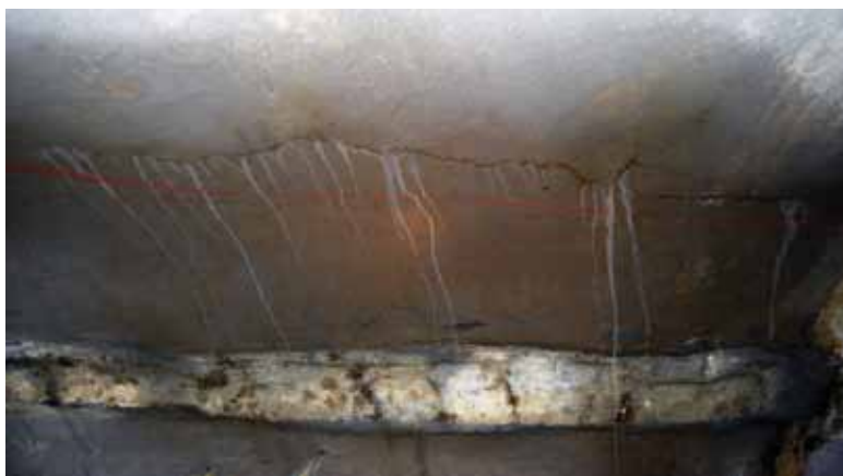
Fig. 3: Water seeping into pipeline
