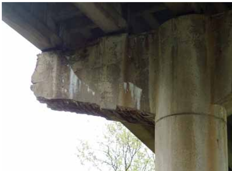
Before repairs, bridge showed major damage due to deterioration
