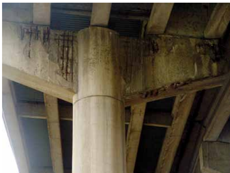
Mid-century bridge in need of repairs
