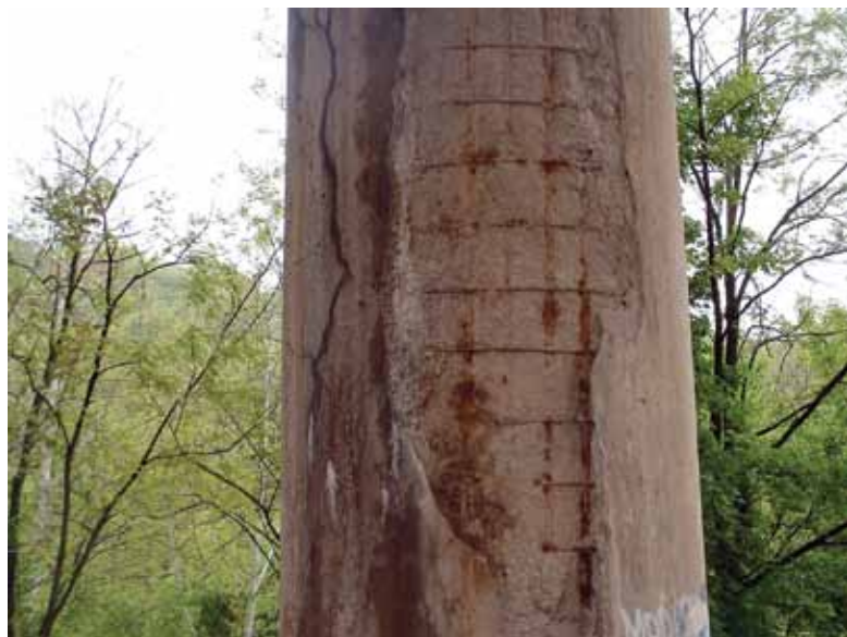
Bridge showed years of deterioration
