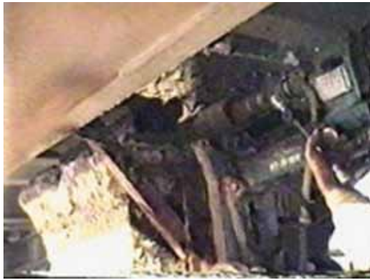
Stitch drilling to separate granite columns from the rest of the structure
