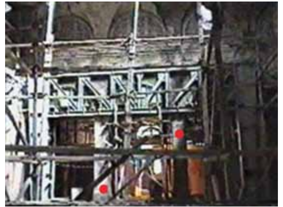
Main truss frame after erection. Granite columns shown before removal, indicated by a dot (●)
