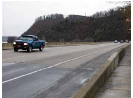
Fig. 8(a): Completed TPCO
