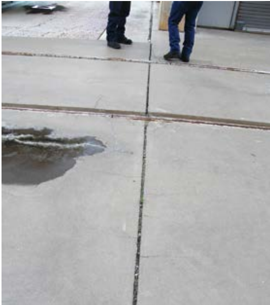
Fig. 3(a): Davis Dam—typical expansion joint before grouting
