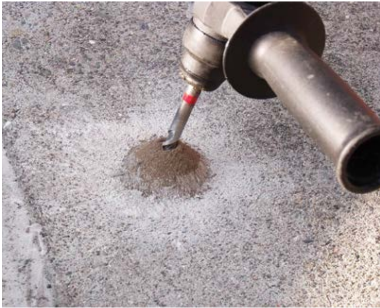
Fig. 7: Drilling holes for injection ports—note color change of cuttings, indicating corkboard has been intercepted
