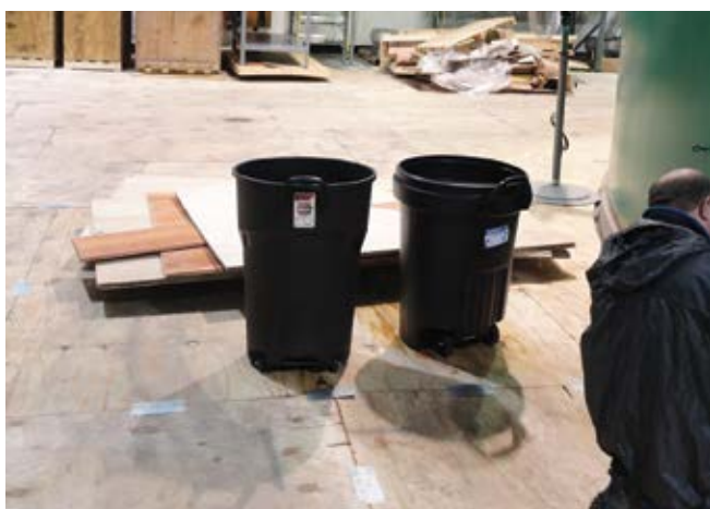
Fig. 1(b): Trash cans used to collect leaking water
