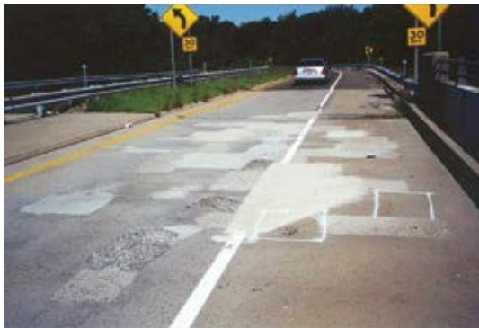
Fig. 4: Deteriorated concrete bridge deck
