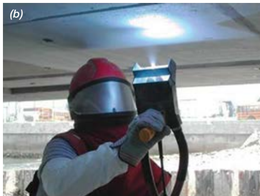
Fig. 9(a) and (b): Port of Canaveral—installation of galvanic protection to piles and concrete deck
