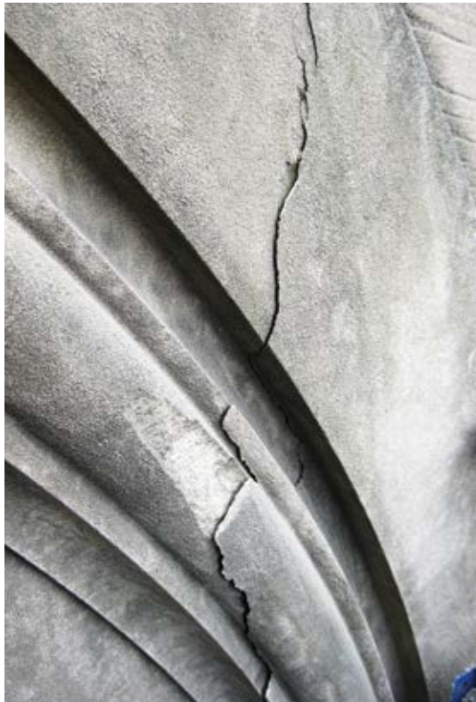
Fig. 6: Severe damage to perimeter unit on right side of “Drama”
