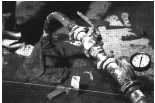
Fig. 7—Typical header setup with wet burlap bag around connection to protect against splatter (Warner 2004).
