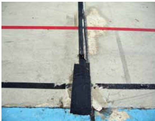
Distressed concrete area at transverse joint—notice the duct tape repairs
