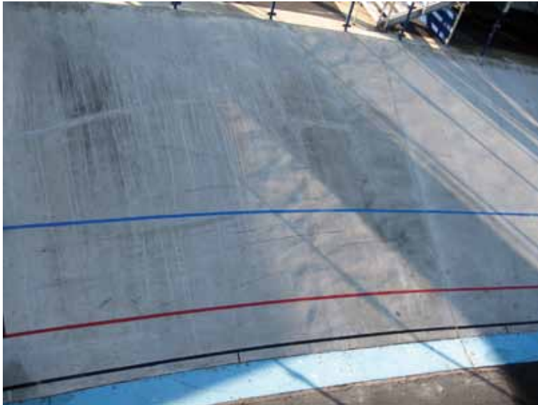
Existing conditions of track surface showed surface deviations (waves on the surface) and discoloration
