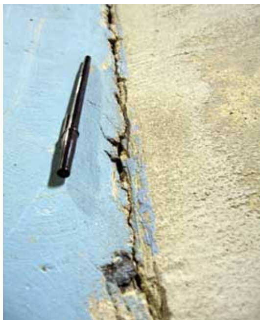
Spalled edges at inside perimeter joint where sloped track meets the interior apron
