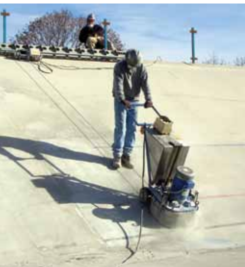
Grinding operation—planetary floor grinder operated on a 30-degree slope, while supported by a custom winch and safety cable assembly
