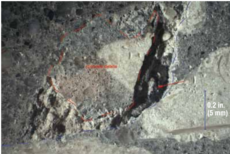
Fig. 6: Large, up to 0.4 in. (10 mm) diameter, concrete debris (outlined in red-dashed line) at contact between deeply recessed, hydrodemolitioned concrete surface and shotcrete repair, separated by blue-dashed line
