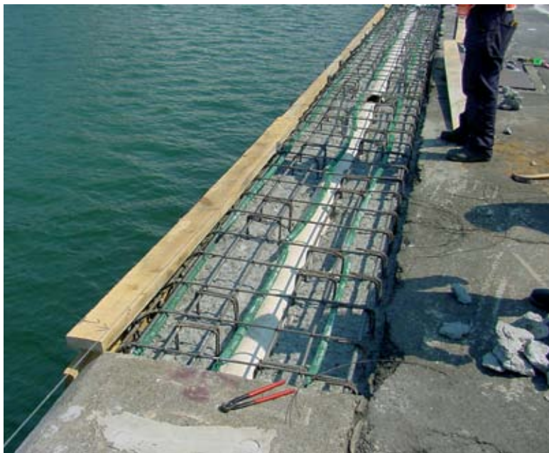
Fig. 8: Monitoring system in place
