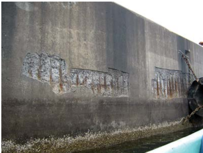
Fig. 2: Damage on the concrete sheet piling crowning beam
