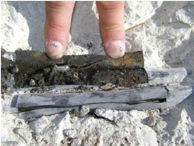
Fig. 2: Exposed strand with severe corrosion and wire section loss for a push-through system
