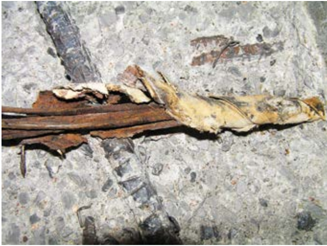
Fig. 1: Paper-wrapped tendon with corrosion deposits
