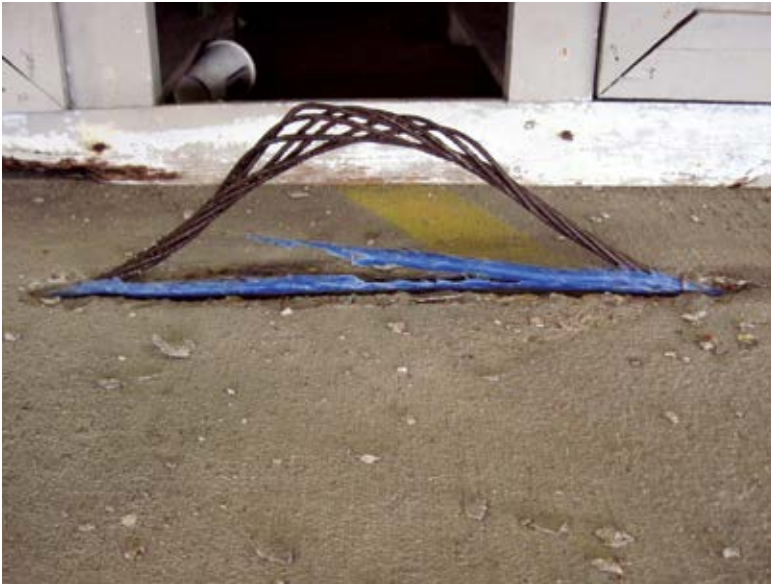
Fig. 6: Post-tensioning tendon failure due to corrosion at high point
