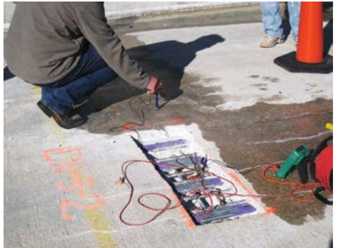
Fig. 4: Corrosion potential testing of mild reinforcement in the vicinity of PT tendons
