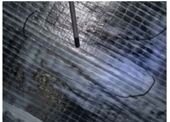
Fig. 12: Delaminated areas identified for repair
