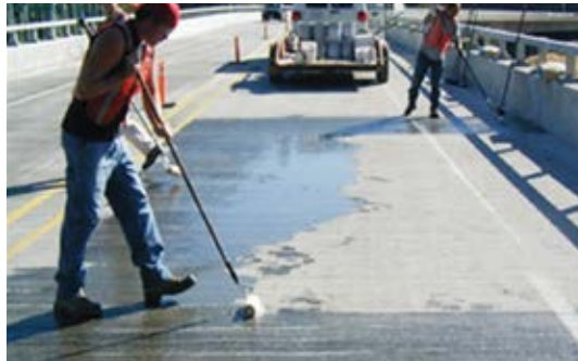
Remove excess epoxy and immediately apply fine sand into the wet epoxy
