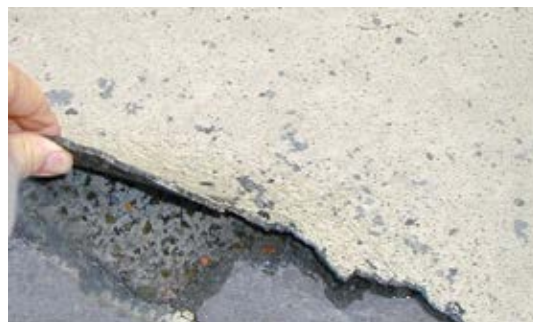
Fig. 2: Protective coating failure
