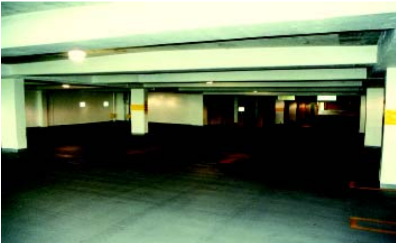
New interior lighting makes brighter driving and parking areas
