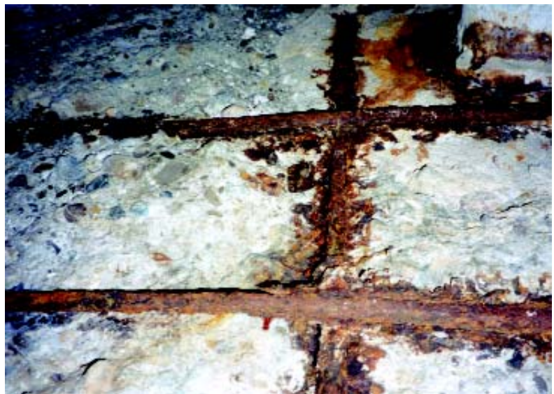
Spalled floor surface
