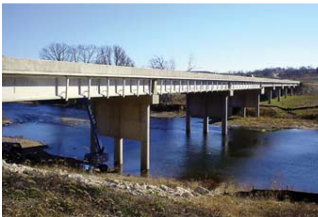
Bridge A5657 on Route 28 over the Gasconade River south of Dixon, Missouri
