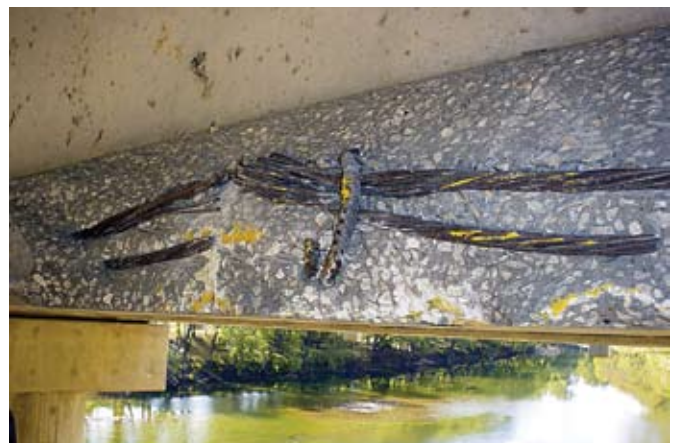
Impact-damaged PC girder of Bridge A5657
