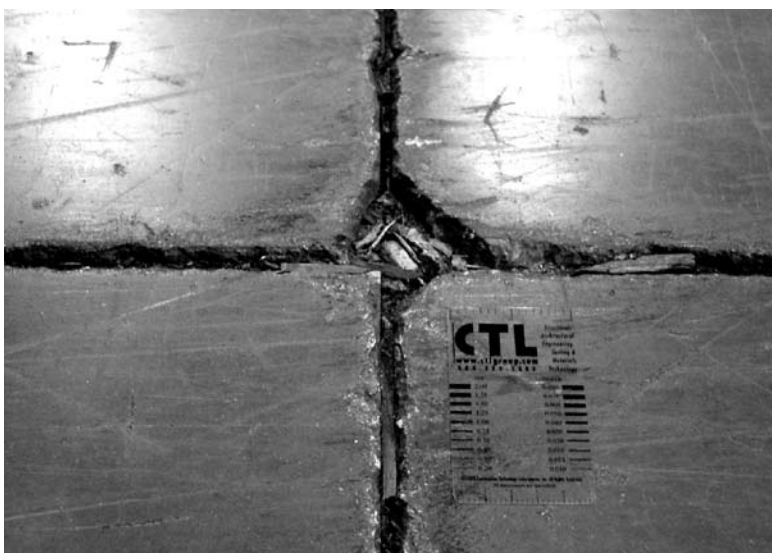
Fig. 2: Severe joint spalling due to lack of early repair
