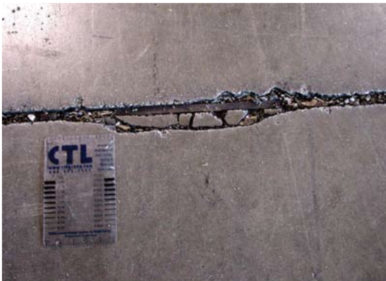
Fig. 1: Joint spalling of an inadequately filled industrial slab joint
