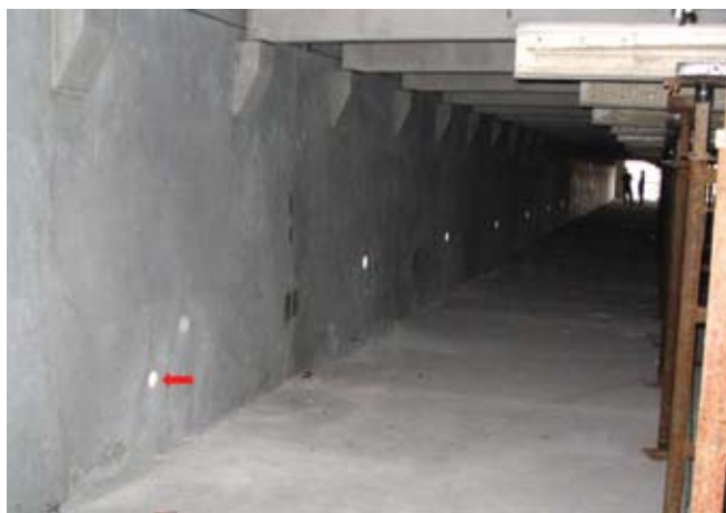
Overall view of typical interior panel faces. Core holes are visible. The inside faces of the panels were generally unaffected by the fire and provided an excellent surface to send and receive impulse signals
