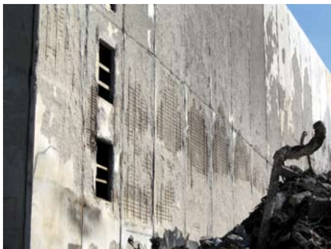
Overall view of portion of the garage where damage was severe and many panels were replaced. Only limited testing was conducted on these panels
