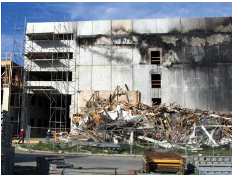
Overall view of garage wall at entrance. Debris is still in place at the time of the site visit, preventing visual inspection of exterior surfaces of lower panels. However, NDT proceeded as planned from the interior surfaces
