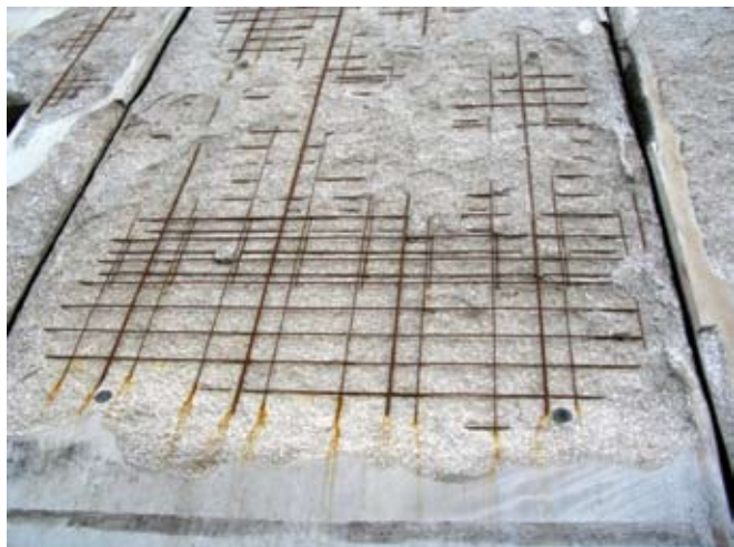
Common degree of damage suffered at the precast panel exterior face due to fire. Spall depths of up to 2-1/2 in. (6 cm) exposing steel were not uncommon
