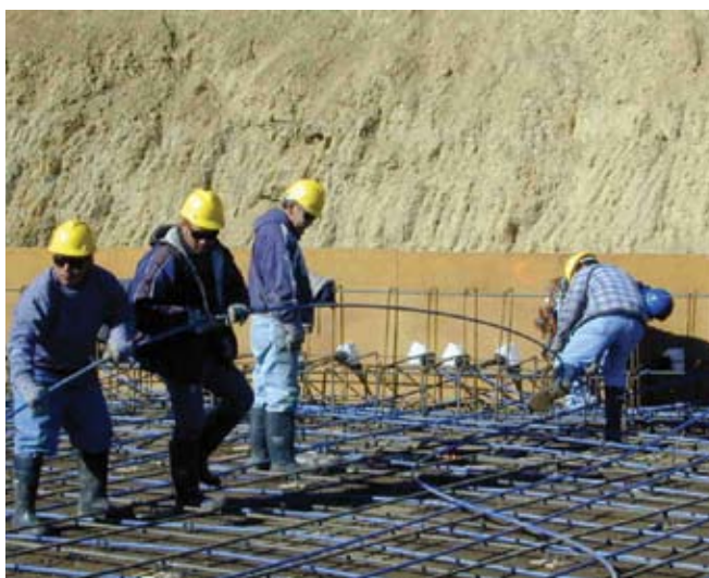
Equipment such as gloves, hard hats, proper footwear, and protective eyewear ensure worker safety
