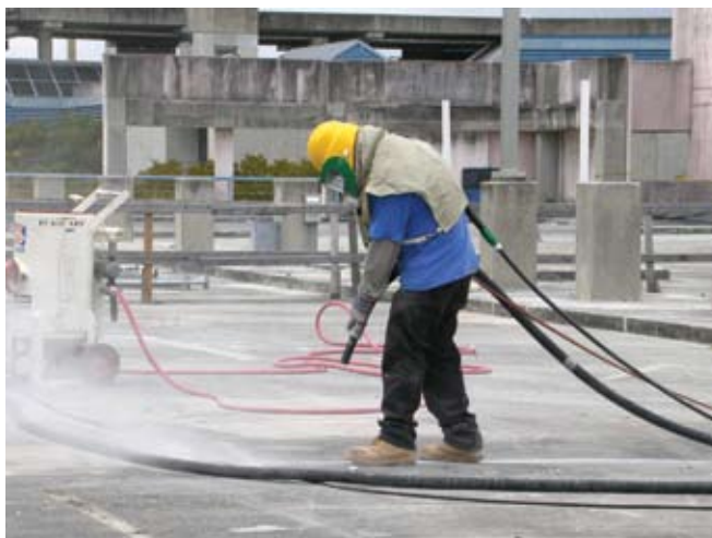
All work must be performed under safe conditions, using the proper protective equipment
