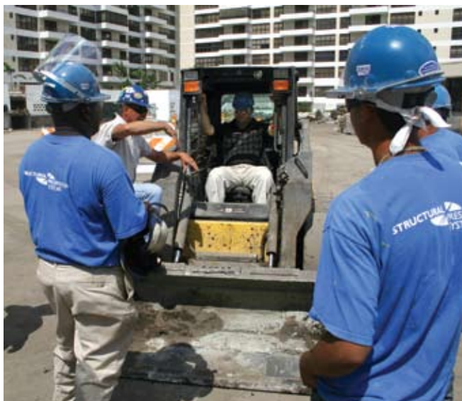
As most repair jobs have unique challenges, site-specific training is also necessary
