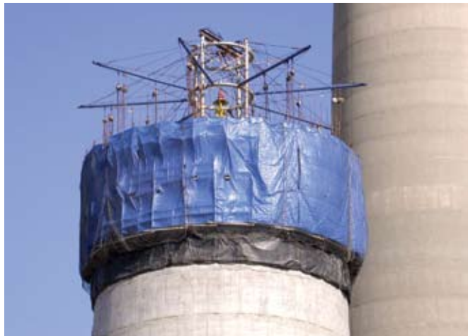
Safety is critical on repair projects, as access is often difficult and potentially dangerous
