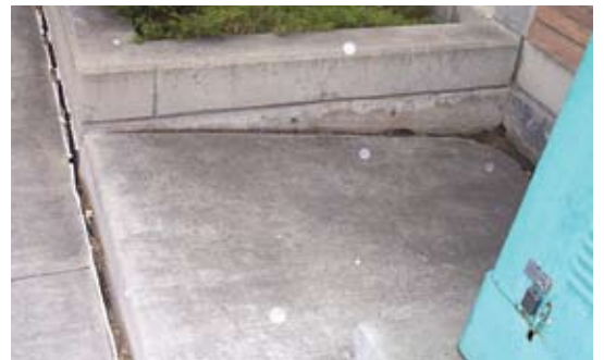
Settling equipment pad
