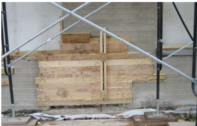
Fig. 5: Formwork in place constructed to match original formboard finish on the existing walls
