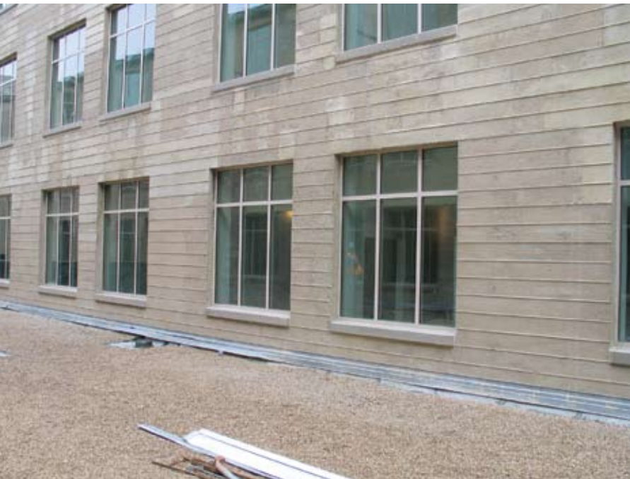
Fig. 6: Portion of wall completed prior to application of silane and potassium silicate coating
