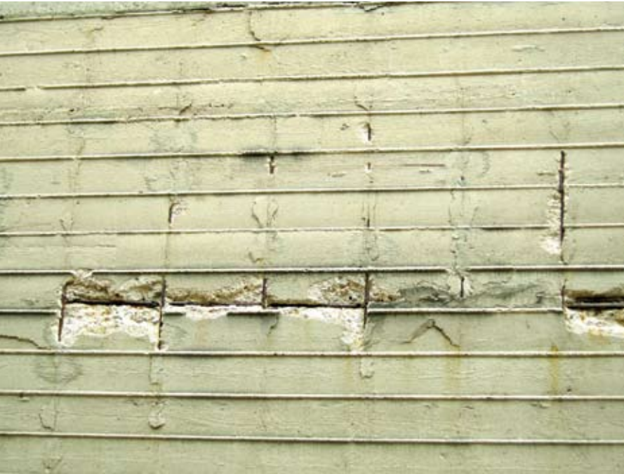
Fig. 1: Typical lightwell wall damage showing spalling and exposed, rusting reinforcing bars
