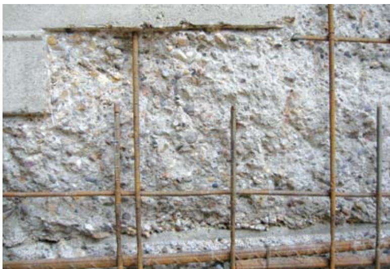
Fig. 4: Close-up view of corrosion-damaged reinforcing bars taken after completion of jackhammer demolition. Note the severe loss of cross section at the bottom of the vertical bars in the photo
