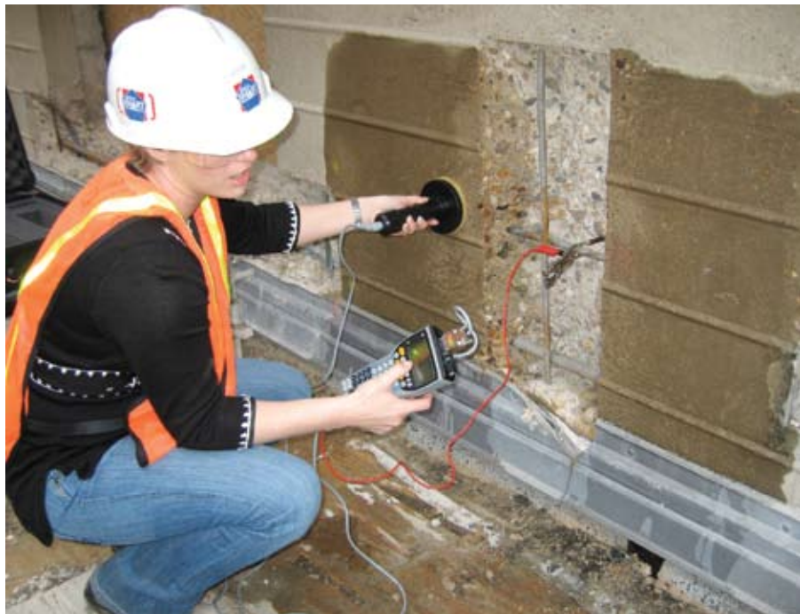
Fig. 8: Corrosion-rate monitoring of corrosion activity in unrepaired portion of wall adjacent to exposed corrosion damage
