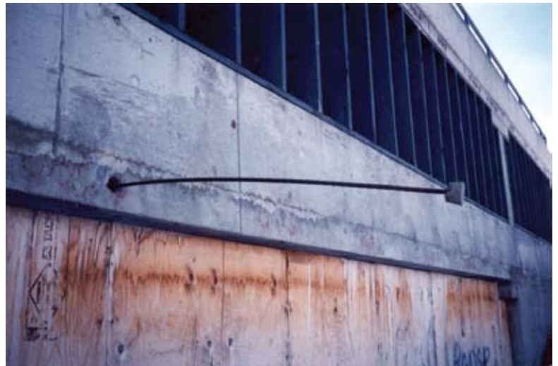
Post-tensioned tendon anchor and grout pocket protruding from parking garage façade after failure
