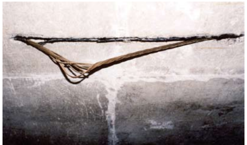
Failed post-tensioned tendon that erupted from slab soffit
