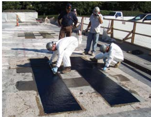
Bonded reinforcement was installed at the top of slab areas around all columns on the elevated levels
