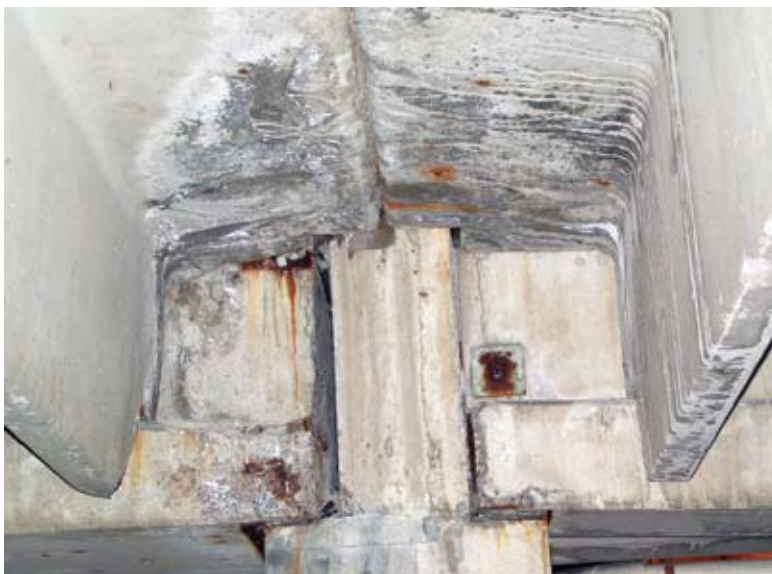
Double-tee deterioration prior to repair
