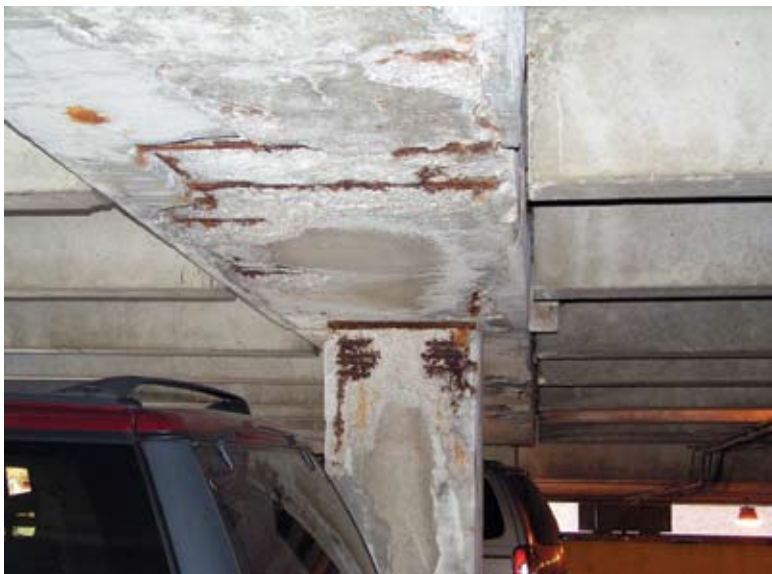
Column deterioration prior to repair
