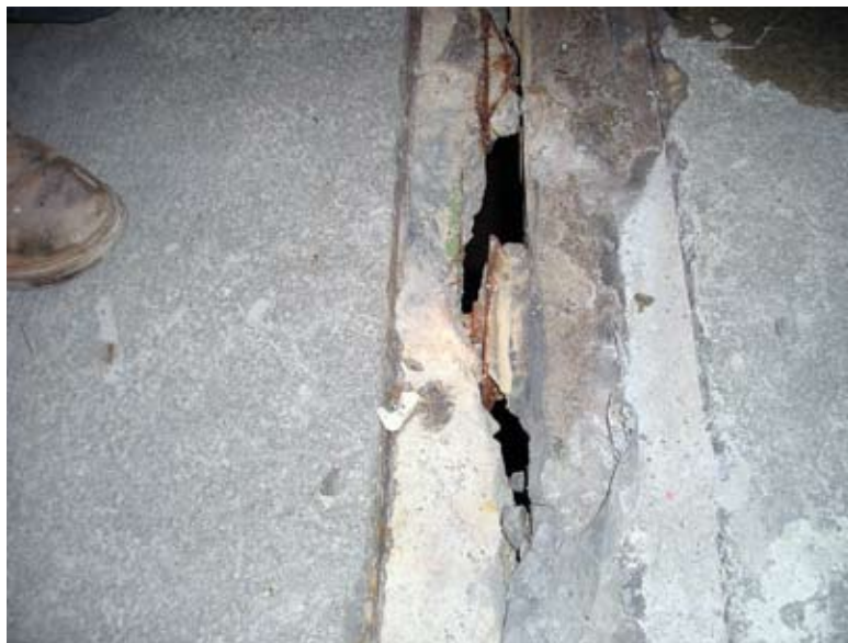
Example of existing conditions of spalled and/or loose concrete present behind existing intermediate anchors
