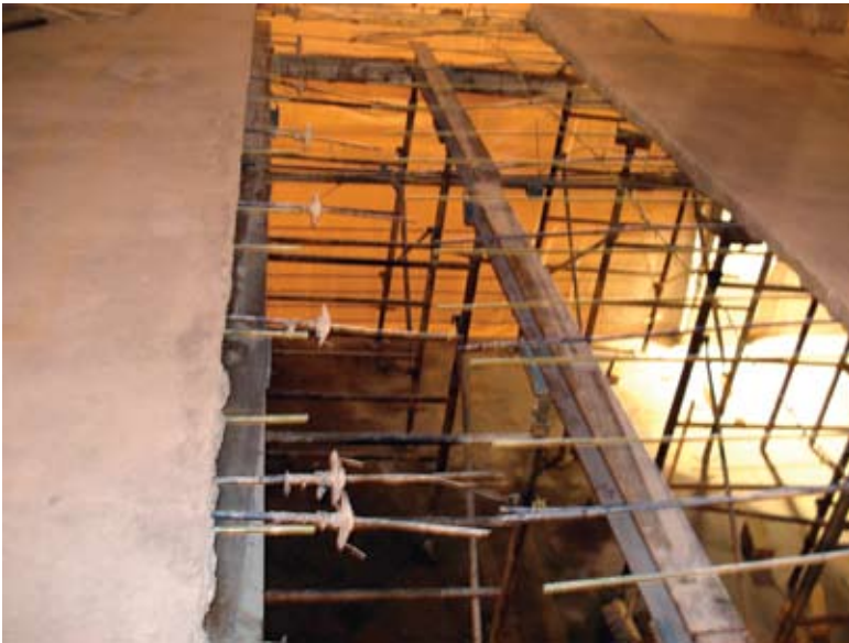
Typical full depth demolition of 6 ft (1.8 m) slab section at the existing intermediate anchors
