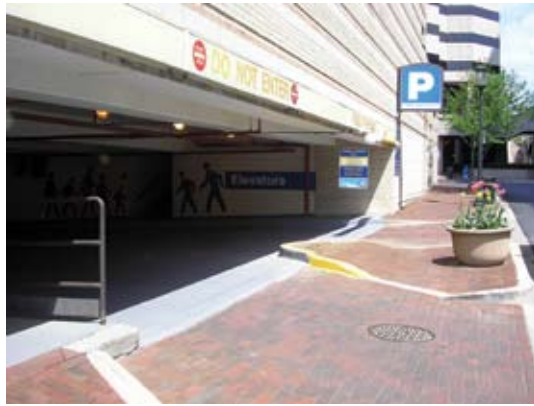
Exterior view of the main garage entrance after the urethane-based waterproofing membrane was applied
