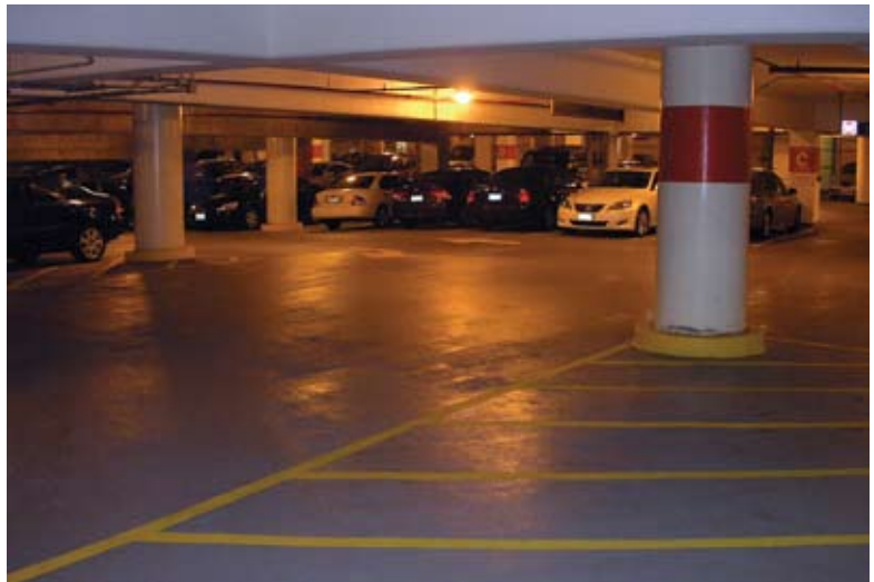
Intermediate parking deck where the urethane-based waterproofing membrane was applied after the post-tensioning repairs were completed
