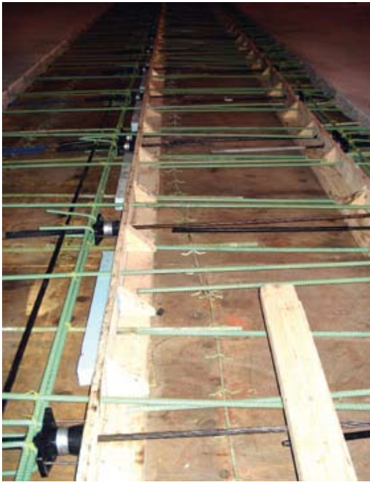
Typical prepour layout of reprofiled tendons, new pour strip and, where necessary, the 1 ft (0.3 m) anchor strip at the location of the previous intermediate anchors
