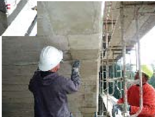
Fig. 5: Use of smooth repair mortar to complete repair. Note recreation of form lines
