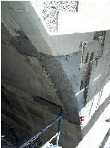
Fig. 4: Deeper repairs held low by 1 in. (2.5 cm) to the surface
