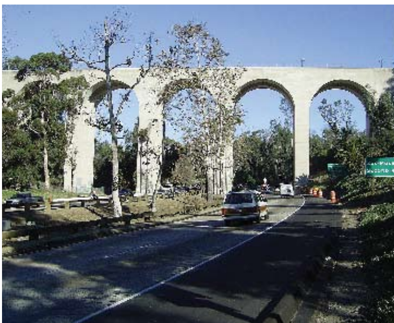
Fig. 6: The Cabrillo Bridge with all historical restoration work complete. Note it does not appear "patched"
