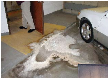
Fig. 2: Ponding and ice near exit
