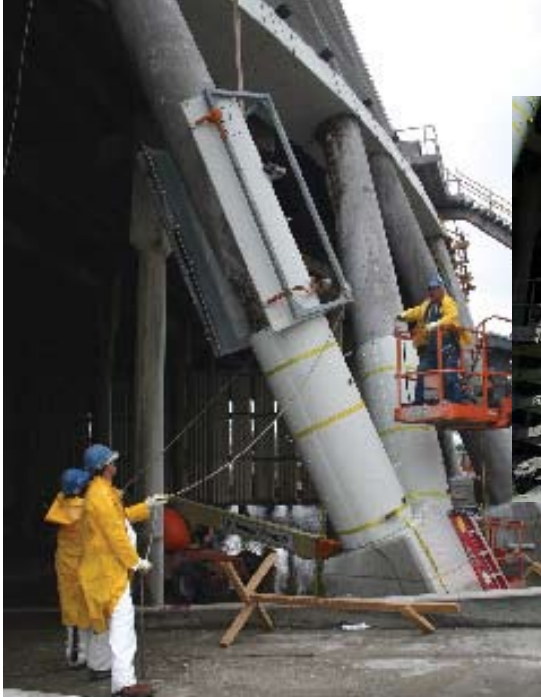
Fig. 4: Jackets for the columns being lifted into place, held open with quick-release straps attached to the lifting bracket
