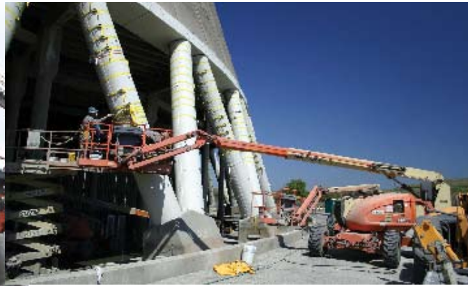
Fig. 5: Ratchet straps being wrapped around each column jacket to increase hoop strength and keep the jacket from warping during grouting
