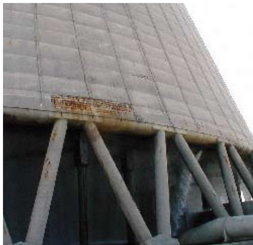
Fig. 2: Corrosion-induced deterioration of the columns and lintel beam
