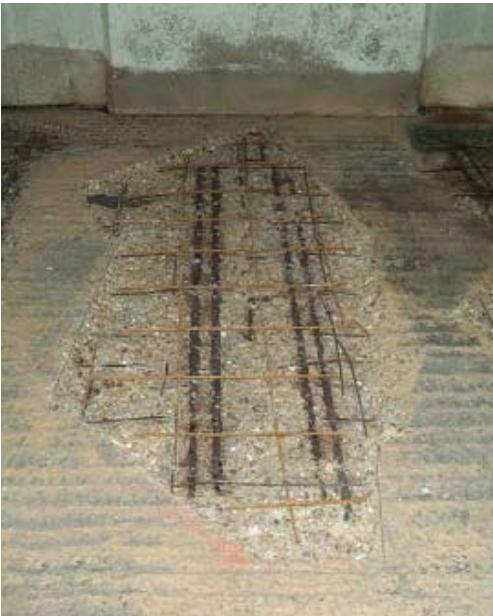
Corrosion of the structure
