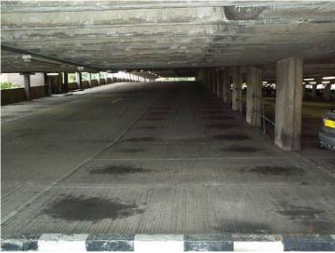
Expansion and day joints were the focal point for growth of the corrosion issues
