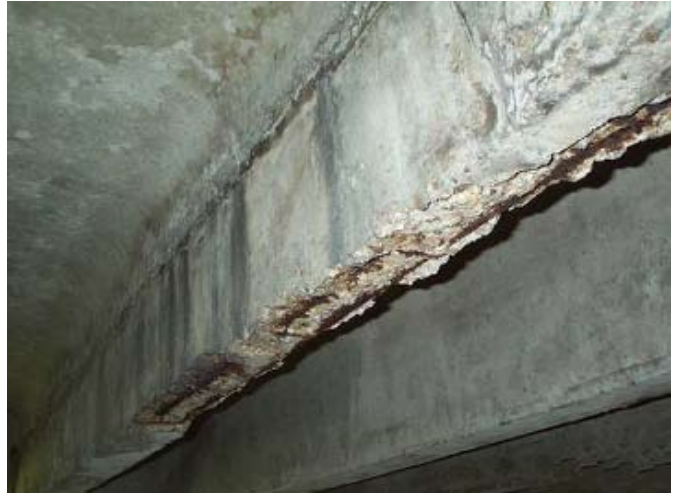
Heavy corrosion was found in some areas
