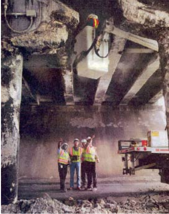
Fig. 2: TXDOT engineers inspect the damage
