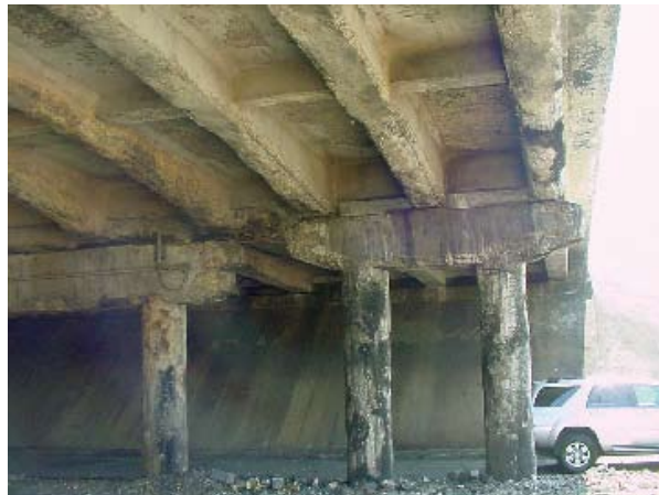
Fig. 1: View looking east of the charred remains of Bent 4 and adjacent areas
