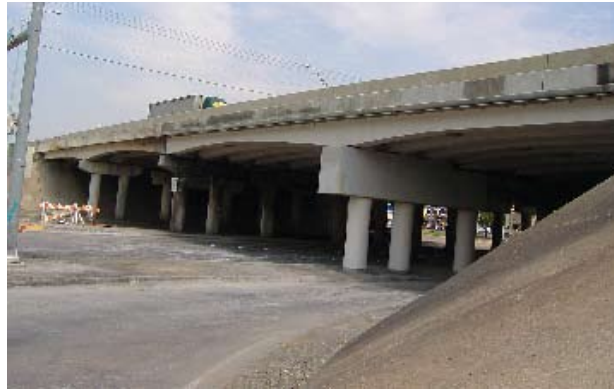
Fig. 6: Completed substructure looking northwest. Bent 4 with the large "straddle" bent is in the foreground
