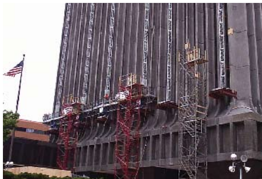
Fig. 5: Mast climbers shown with the 40 ft (12.2 m) high stair access towers from the plaza level
