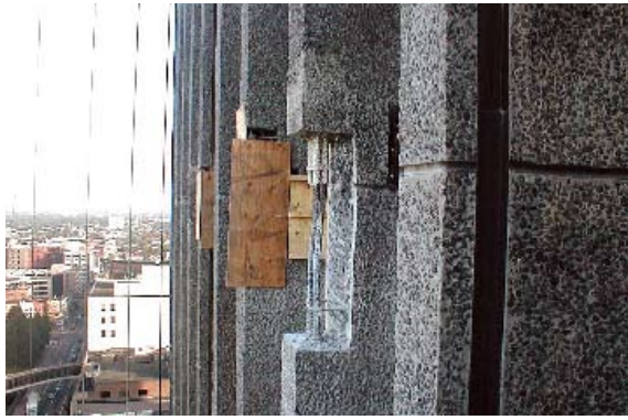
Fig. 2: Typical location of deteriorated concrete after demolition
