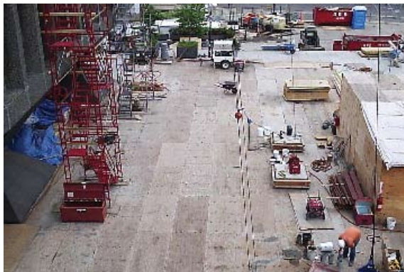
Fig. 4: The entire plaza area was fenced and covered with a flooring system to protect the paver system
