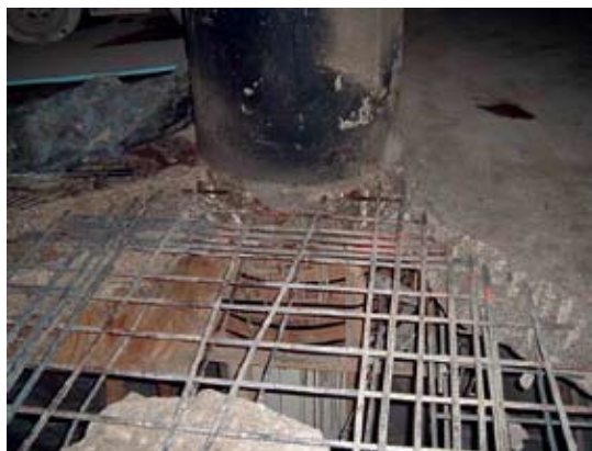
Sequencing of full slab removal of column with 46 stories above it. The slab removal was done in four quadrants. Note shear collar at top of columns added to reestablished shear
