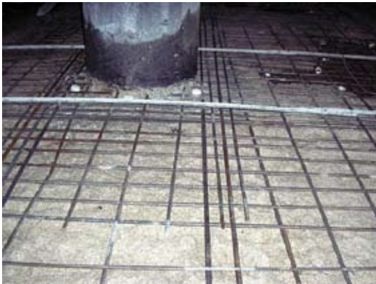
Anodes have been placed to mitigate the halo effect. Note that the additional top reinforcement has been placed around the column to meet current code requirements
