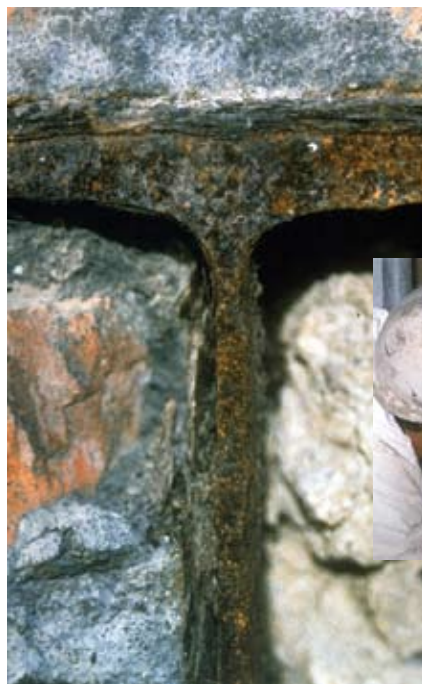
View of steel frame with diminished cross section to the flange and web and demonstrating exfoliated rust layers
