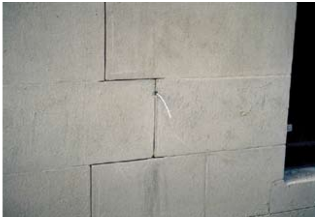
Installation of discrete anodes complied with conservation policy and the principle of "minimum intervention"
