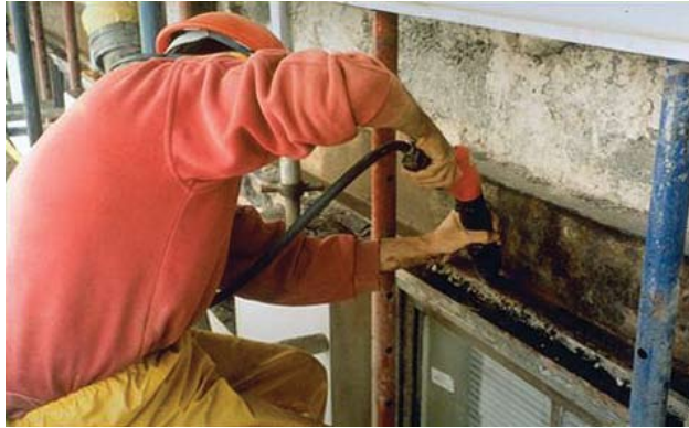
Labor-intensive preparation by needle gunning corrosion product from deconstructed sections of the façade
