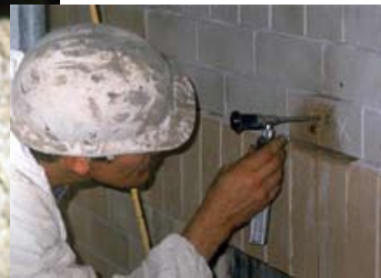
Using anode drill holes to perform final inspection for voiding with bore scope
