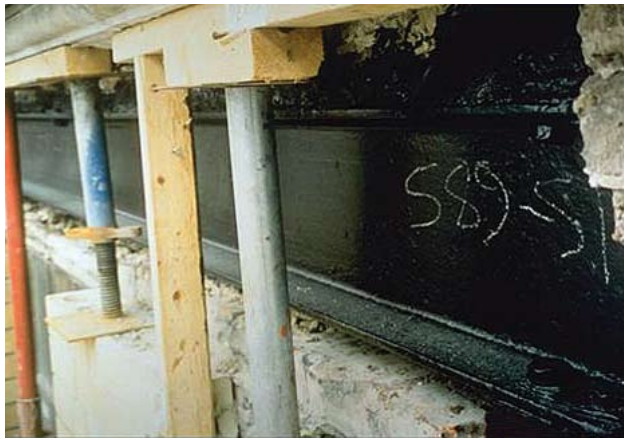
Following prime coat, a final high build coat is applied prior to rebuilding the façade
