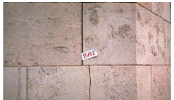
Aesthetic deterioration caused by the cracking of the stonework
