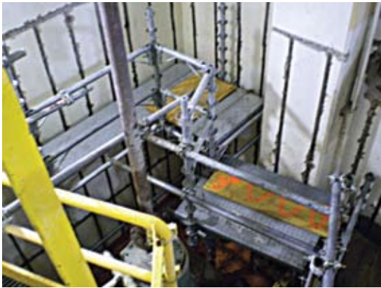
Intricate scaffolding required to cut slots and perform concrete demolitions in SWPs
