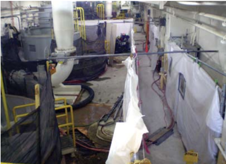
The setup of the protective area demonstrated the phasing and challenges of all the equipment that had to be worked around
