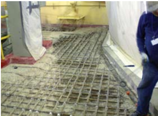
Anodes were attached with zip ties to a nonconductive spacer to keep it off the reinforcing steel, preventing shorting of the system
