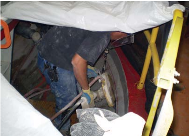
Saw cutting of slots in CWB. Tight quarters made planning of the work critical to the success of the project
