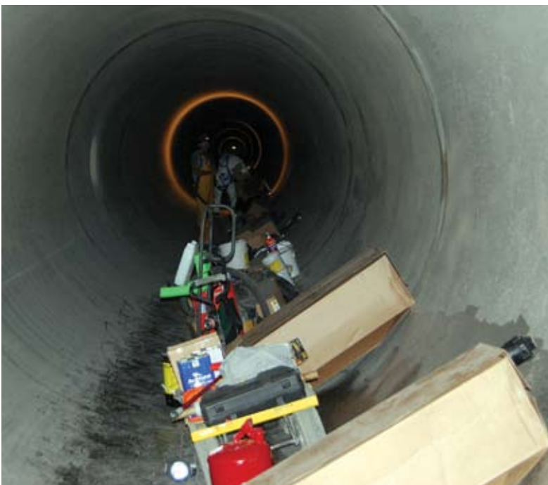
Materials were spaced out throughout the 840 ft (256 m) long section of pipe
