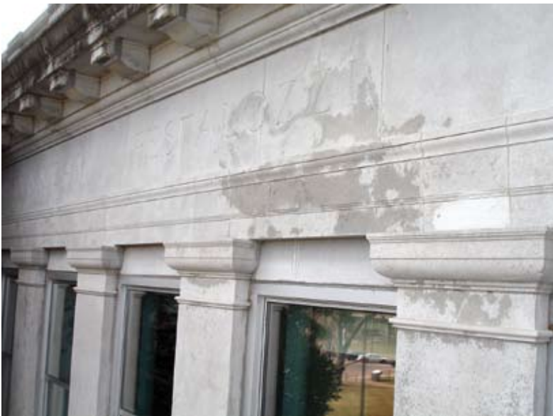
Deterioration and discoloration of stone on Hill Hall
