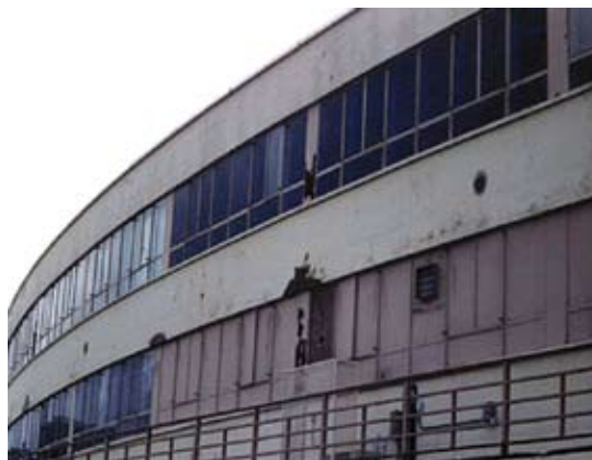
Damage included cracking, spalling, and reinforcing steel corrosion
