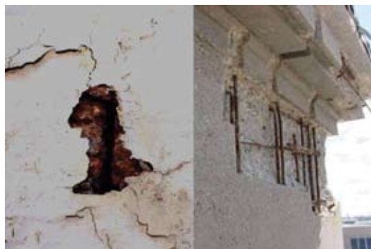
Typical corrosion condition before and after concrete removal
