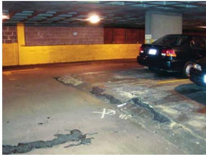
Deteriorated concrete overlay with trip hazard
