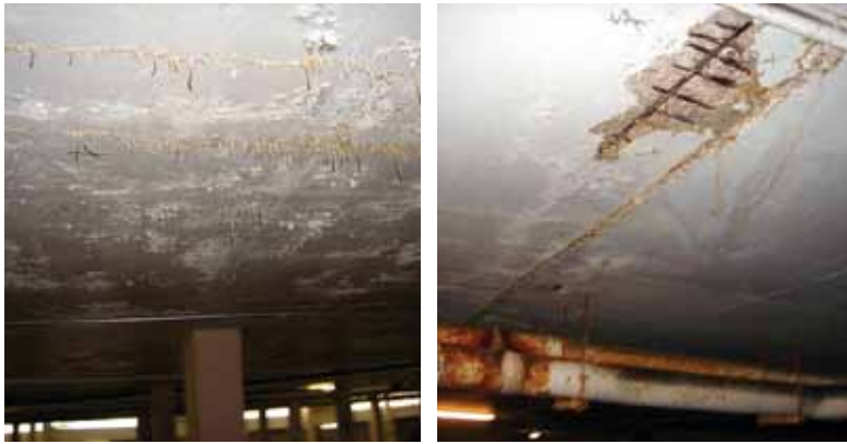
Deterioration prior to repair
