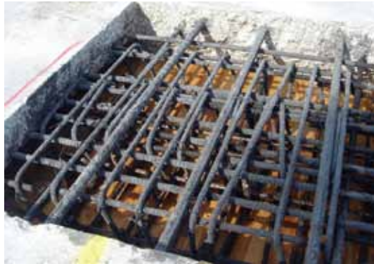
Congested steel reinforcement
