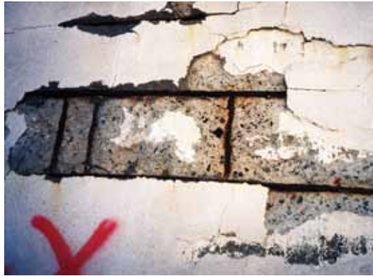
Fig. 1: Area showing severe deterioration, marked for concrete removal
