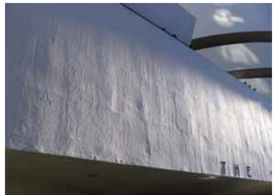
Guggenheim Museum's Fifth Avenue façade showing coating failures before repair work
