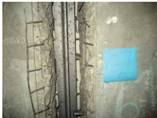
Exposed sixth floor 2-1/2 x 2-1/2 in. (63.5 x 63.5 mm) steel tee after abrasive cleaning
