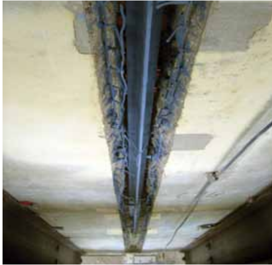
Remedial control joint at sixth floor tee location
