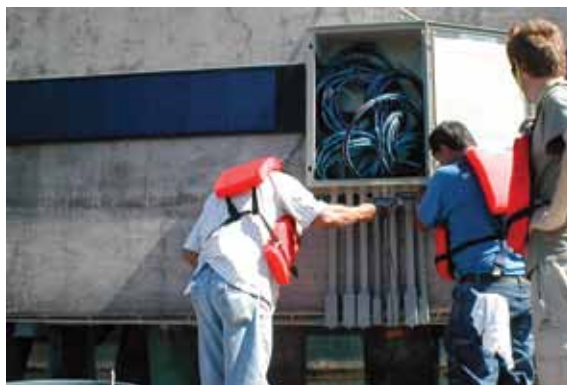
Installation of remote monitoring system on dolphin platform face. Note the solar panel used to provide energy needed to run wireless communications
