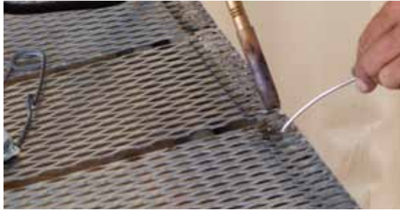
Zinc mesh panels were cut to fit each face of the octagonal pile and connected by soldering a zinc strap at the top of the panels prior to placement on the piles
