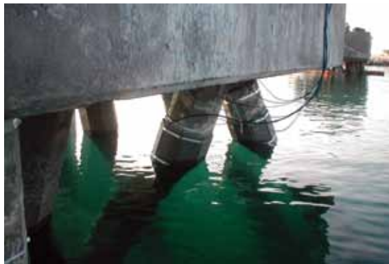
Wiring has been connected to the anodes, testing instruments, and reinforcing and awaits placement in conduits and termination at control boxes
