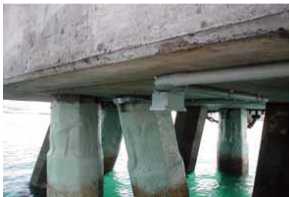
Completed jackets and conduit for wiring
