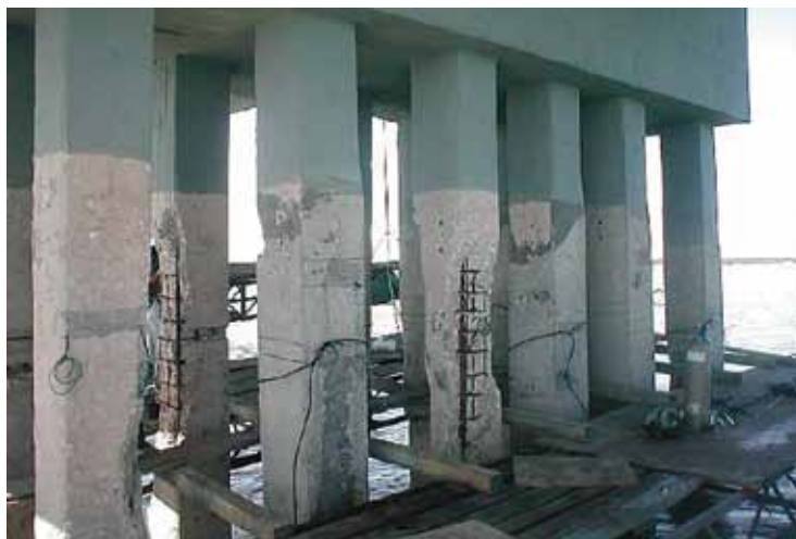
Bent cap with metalized cathodic protection system installed and pilings prepared for Lifejacket System
